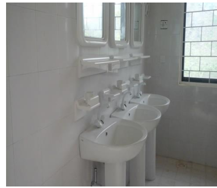
Sanitary fixtures in bath room
