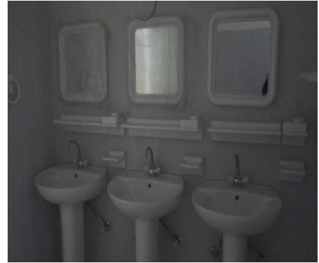
Sanitary fixtures in bath room
