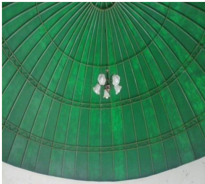
Seepage observed along the dome inner sides
