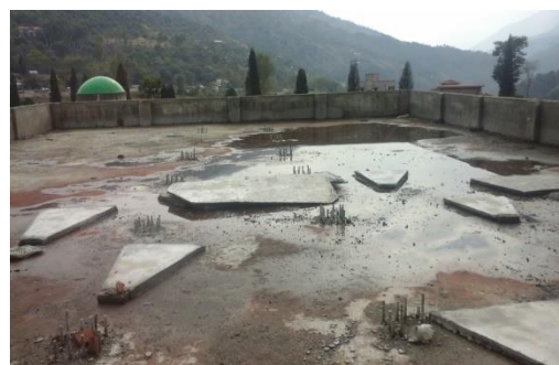
Steel reinforcement of top floor columns left opened not following the engineering standards
